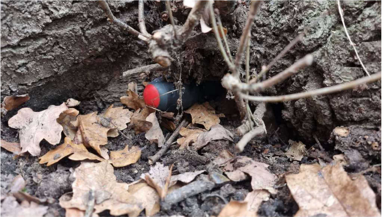
T1 oak photo 1 - Screwdriver inserted into the decay at the base between the buttress roots on the south side
