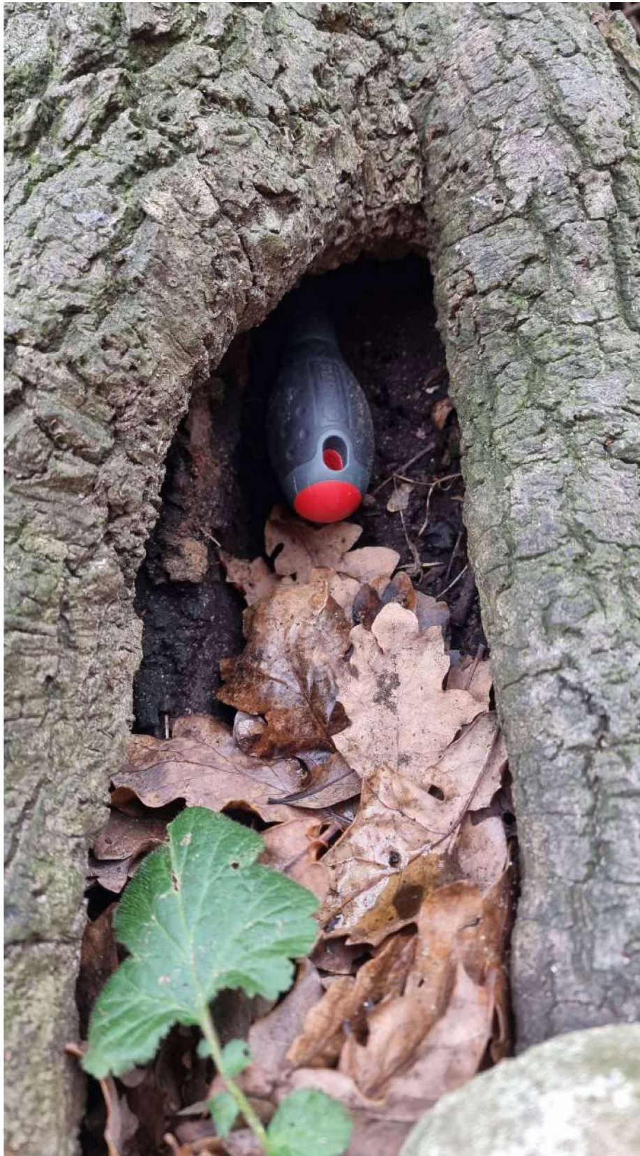
T1 oak photo 2 - Screwdriver inserted into buttress root cavity on the south side
